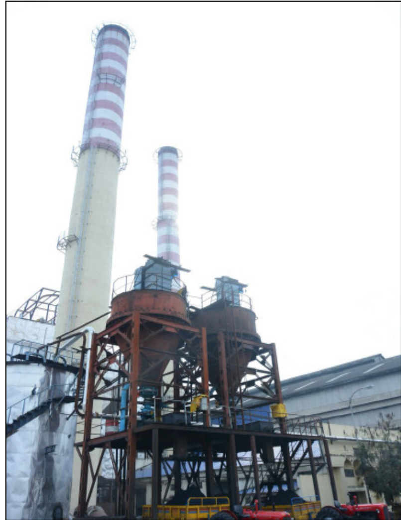
Boiler Ash Handling System
